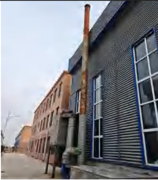
15m 排气筒 DA001
