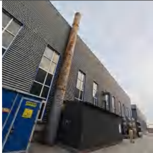
15m 排气筒 DA002
